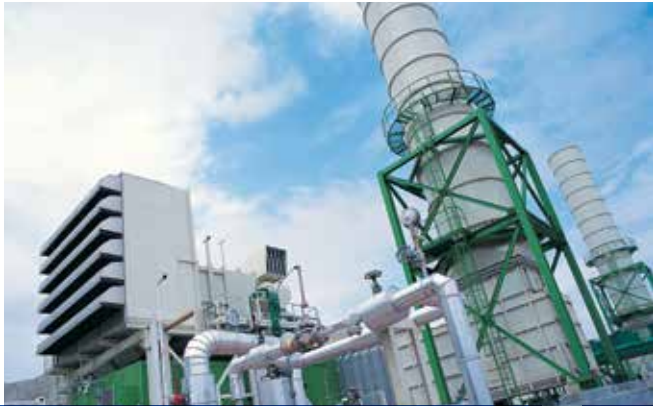
Turkmenbashi Refinery Simple Cycle Power Plant
