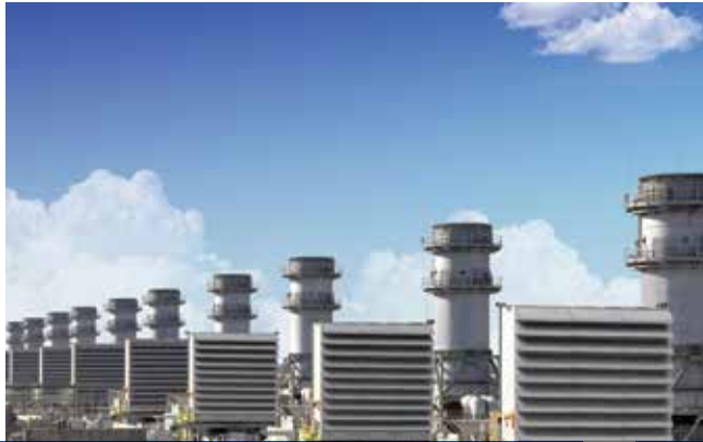
Al-Khairat Simple Cycle Power Plant
