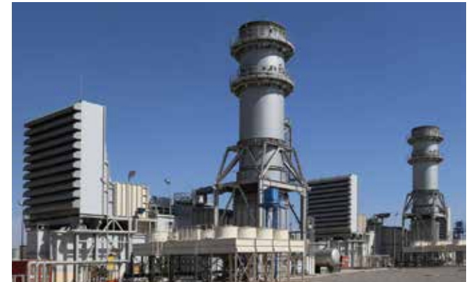
Bazian Combined Cycle Power Plant
