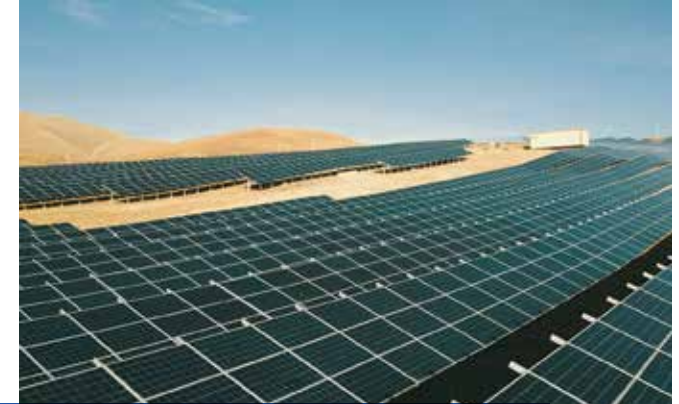
Erzurum Solar Power Plant
