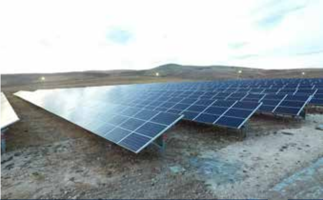
Polatlı Solar Power Plant
