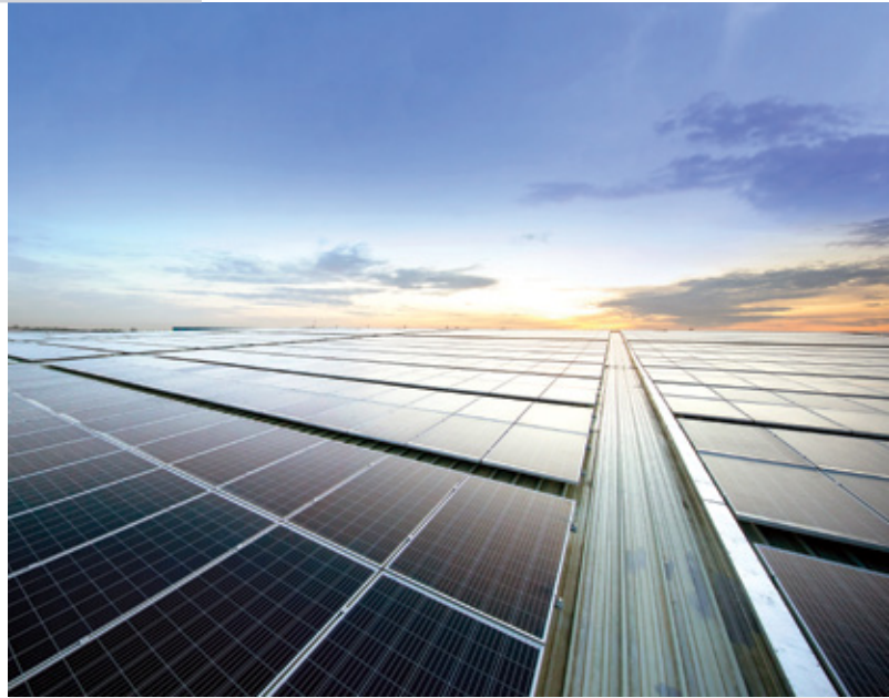
→ Solar panels installed at our Singapore aerospace facilities help fulfil 30% of our electricity needs
