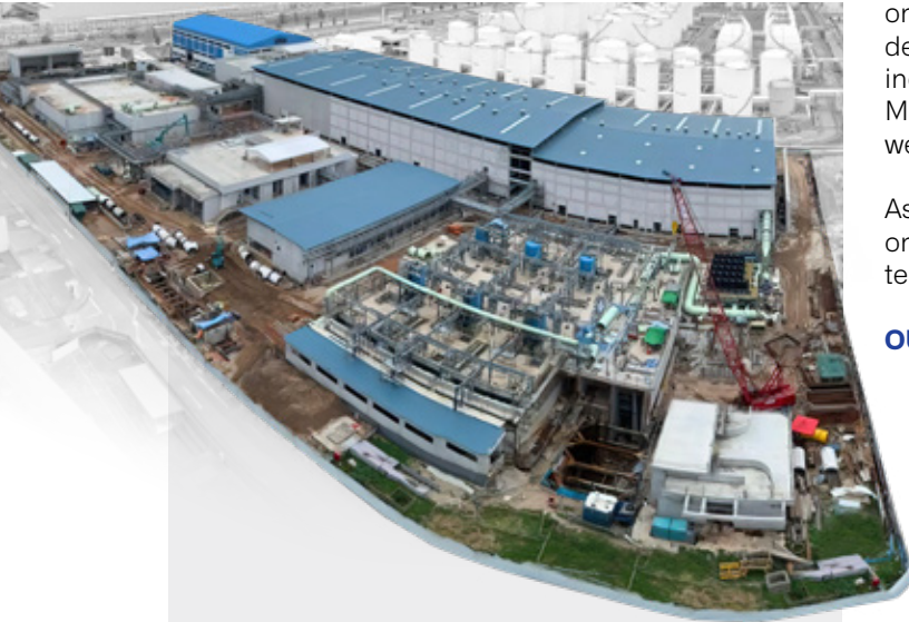
→ An aerial view of the Jurong Island Desalination Plant which is expected to be completed in 2022. This will be Singapore's fifth desalination plant.
