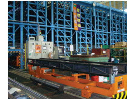
The automated rack stocker for storage of long pallets
