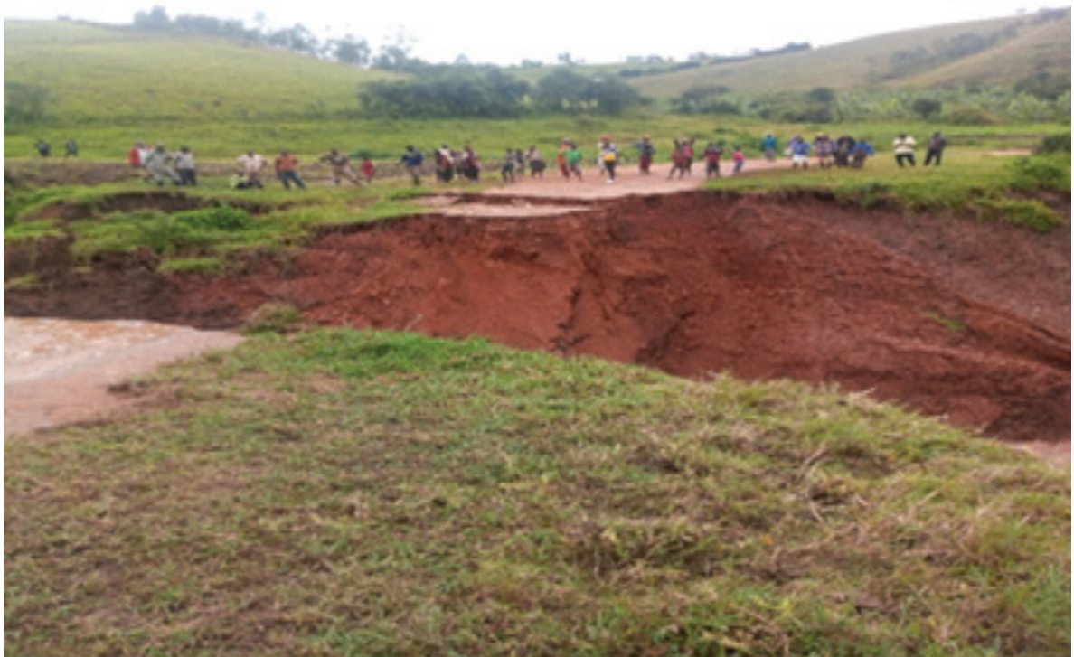
Figure 6: Caved in road sections along Kabale-Ntungamo (above) and Rwashamaire Rwahi (below)
